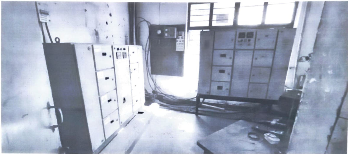
Electric Sub-station Block-2
