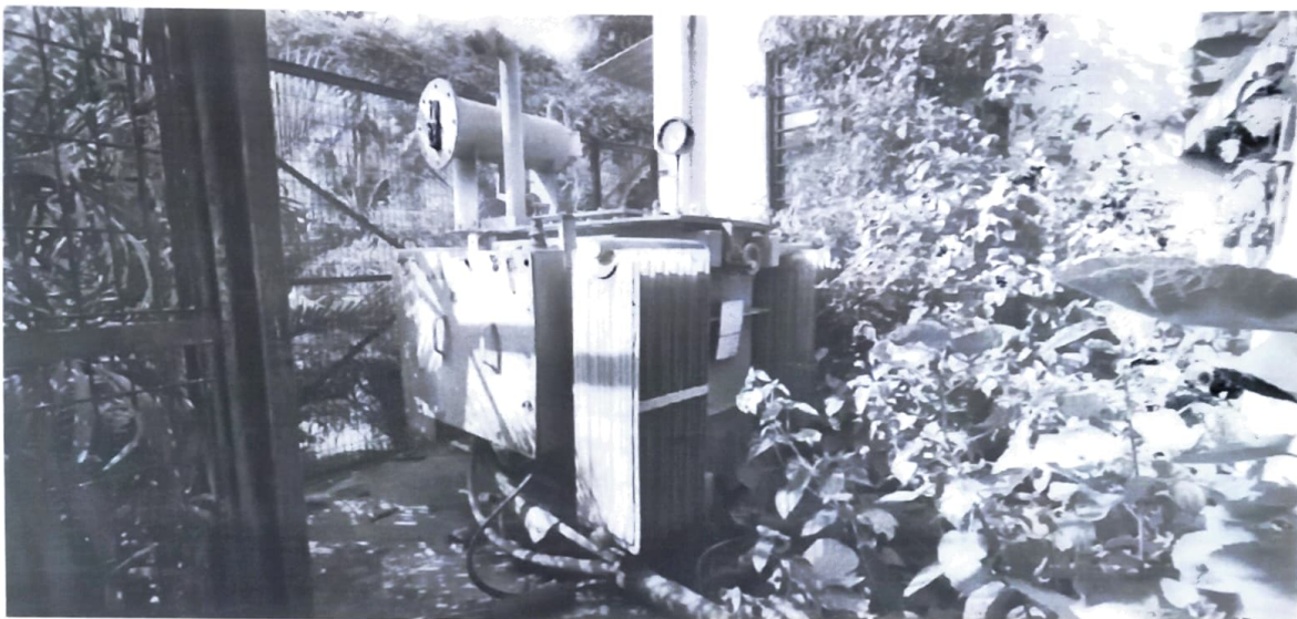
Transformer at Sub-Station
